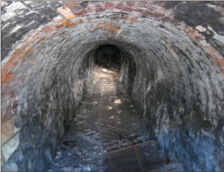
One of the tunnels below the Doncaster to Sheffield railway line at Levitt Hagg.
